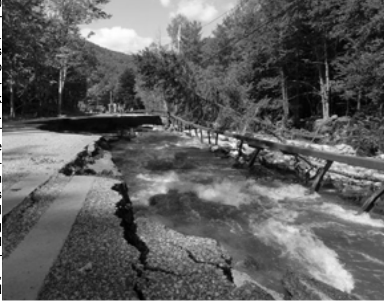
A road in Southern Vermont Flooded by Hurricane Irene
